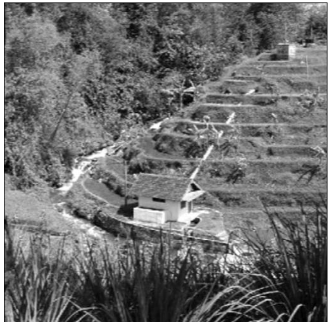
A micro-hydro power penstock carrying water through terraced ricefields to the powerhouse (Seloliman, East Java, Indonesia).
